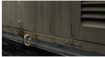
Figure 4: The condensate pipe draining from the DX cooling coil, fitted with P-trap/U-bend
