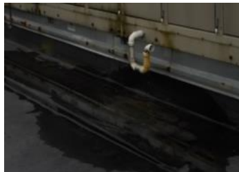
Figure 5: The lack of appropriate drainage methods adjacent to AHU curbing beneath condensate pipe
