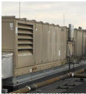
Figure 3: One of nine (9) rooftop air handling units (AHU)
