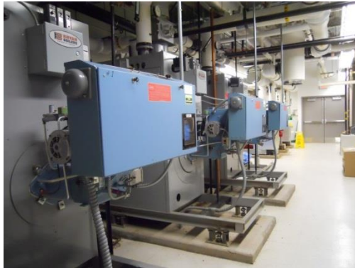
Figure 2: The boilers, located in the Mechanical Room, which feed the Institute of Rehabilitation
